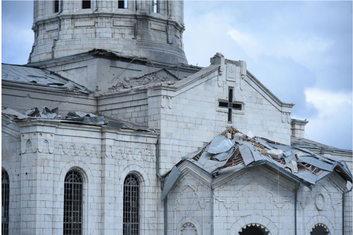
Some of the damage caused to Ghazanchetsos Cathedral in Shushi.
