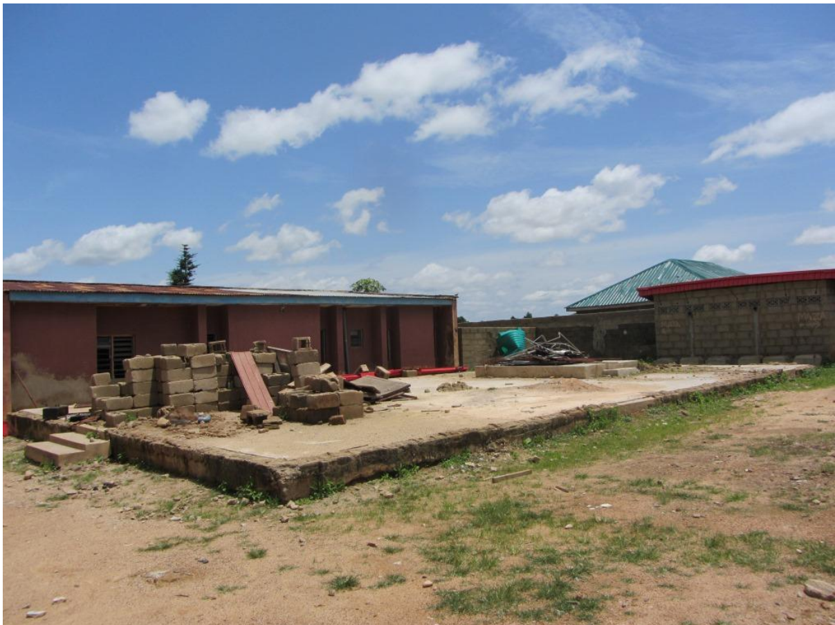
Destruction of Children's Meeting Hall, ECWA Church, Wasasa, Kaduna State.
