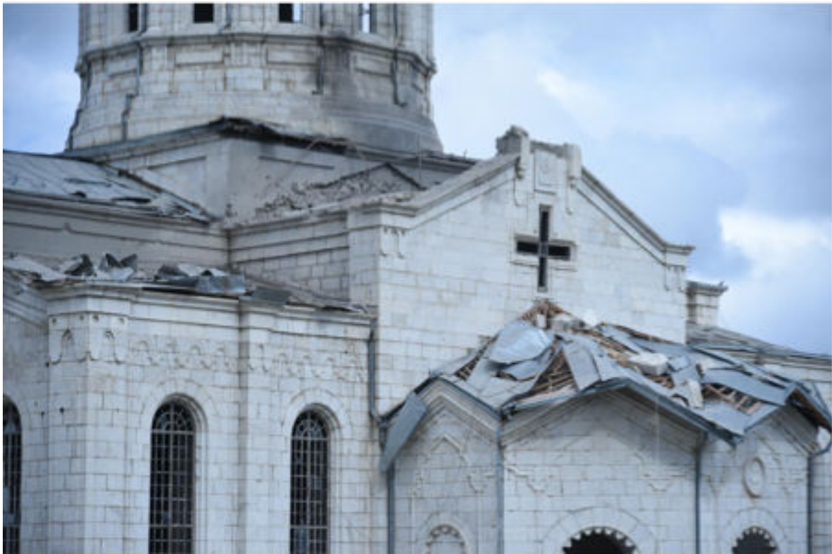
Some of the damage caused to Ghazanchetsots Cathedral in Shushi on 8 October 2020.
