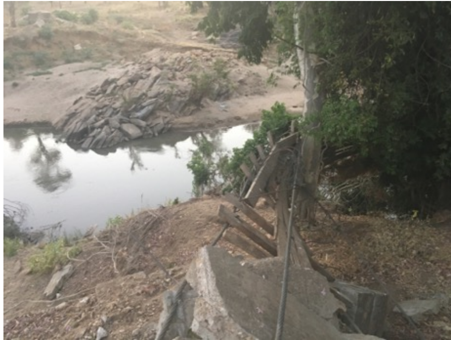
Figure 2 Wooden footbridge swept aside, August 2017
