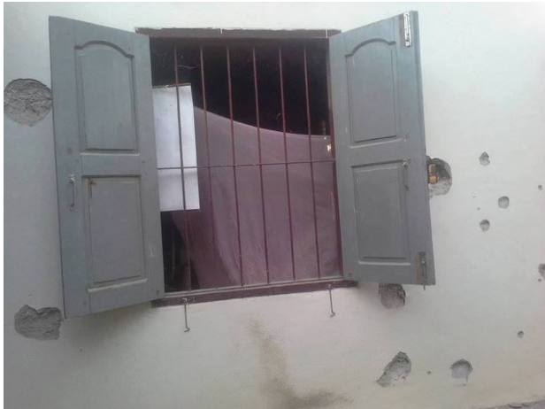
Shrapnel damage at Nang Kaeng's house
